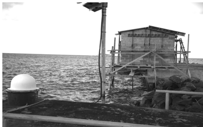
Fig 1: Building to house new tide gauge as part of the Indian Ocean Tsunami Warning System
